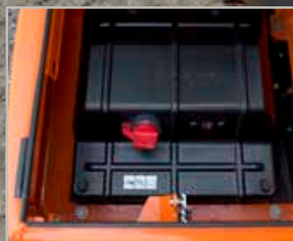
Battery cut-off switch
